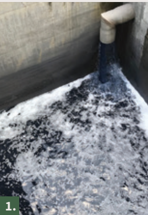
1. Water from the dye house enters the system.
